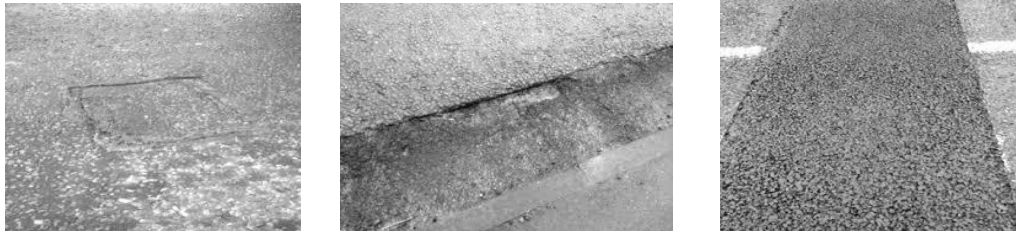
Fig. 15. Effect of low and non-uniform compaction - deployment of the seal starting with perimeter areas.
