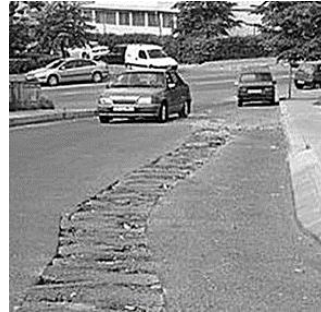
Fig. 19. Poor repair of road infrastructure after utilities' interventions.
